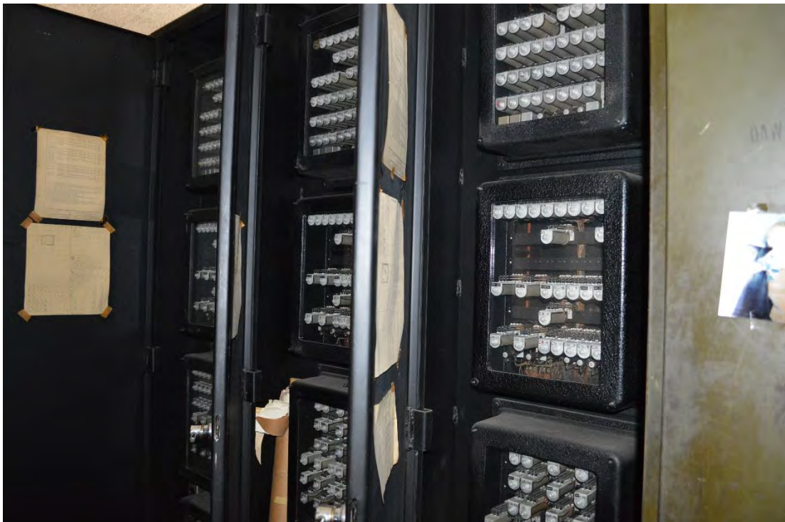
Photograph 16: Detail of General Electric Equipment Cabinets.
