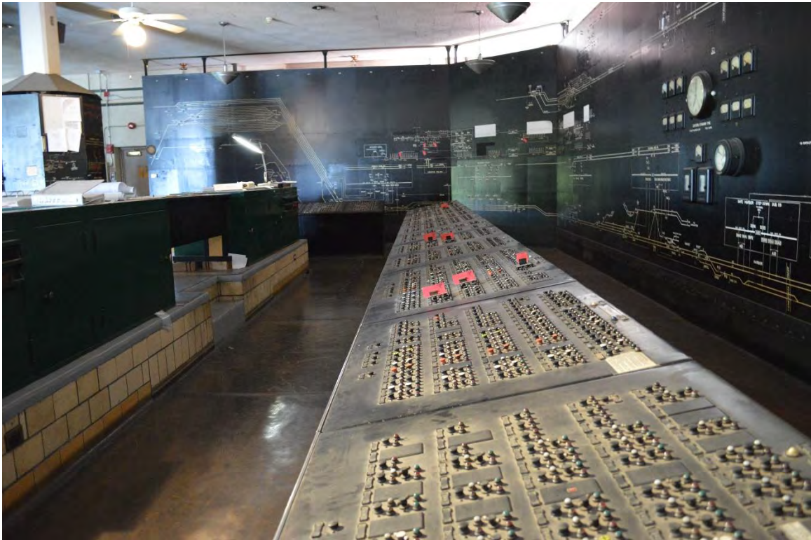
Photograph 9: Westinghouse twelve-panel console.
