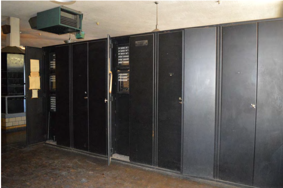
Photograph 15: Detail of General Electric Equipment Cabinets.
