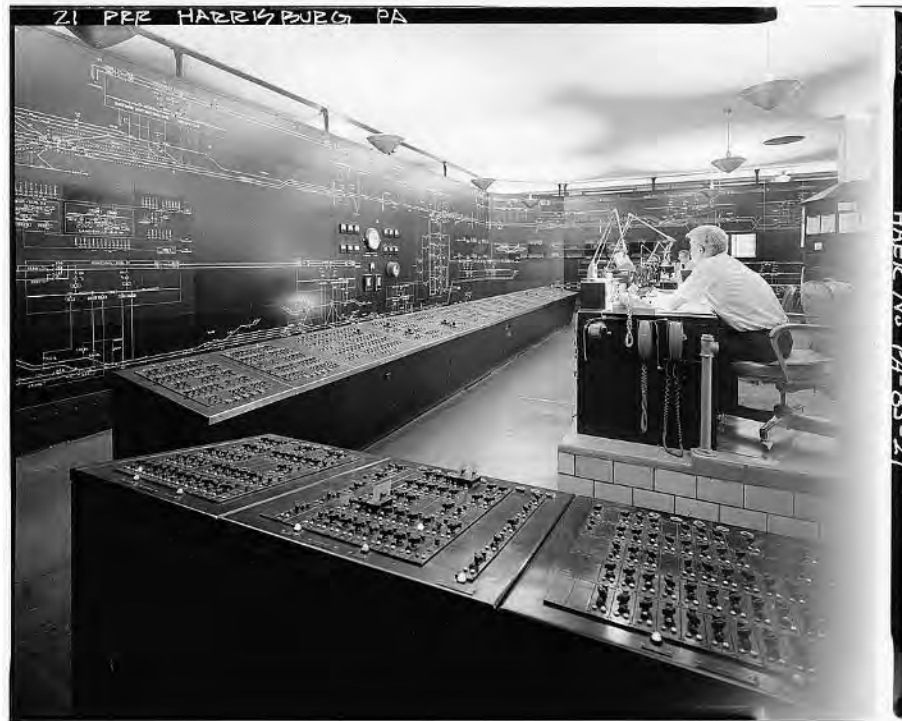
Image 29: Interior view of power directors room, second floor (this is the control center for direction of electric power for trains across the state). Note display boards. (HAER 1985)
