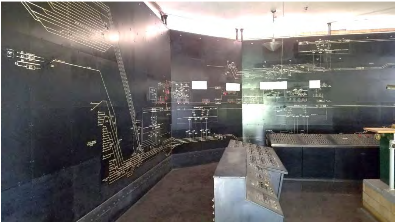
Image 32: Interior view of power directors room, second floor, 2017.
