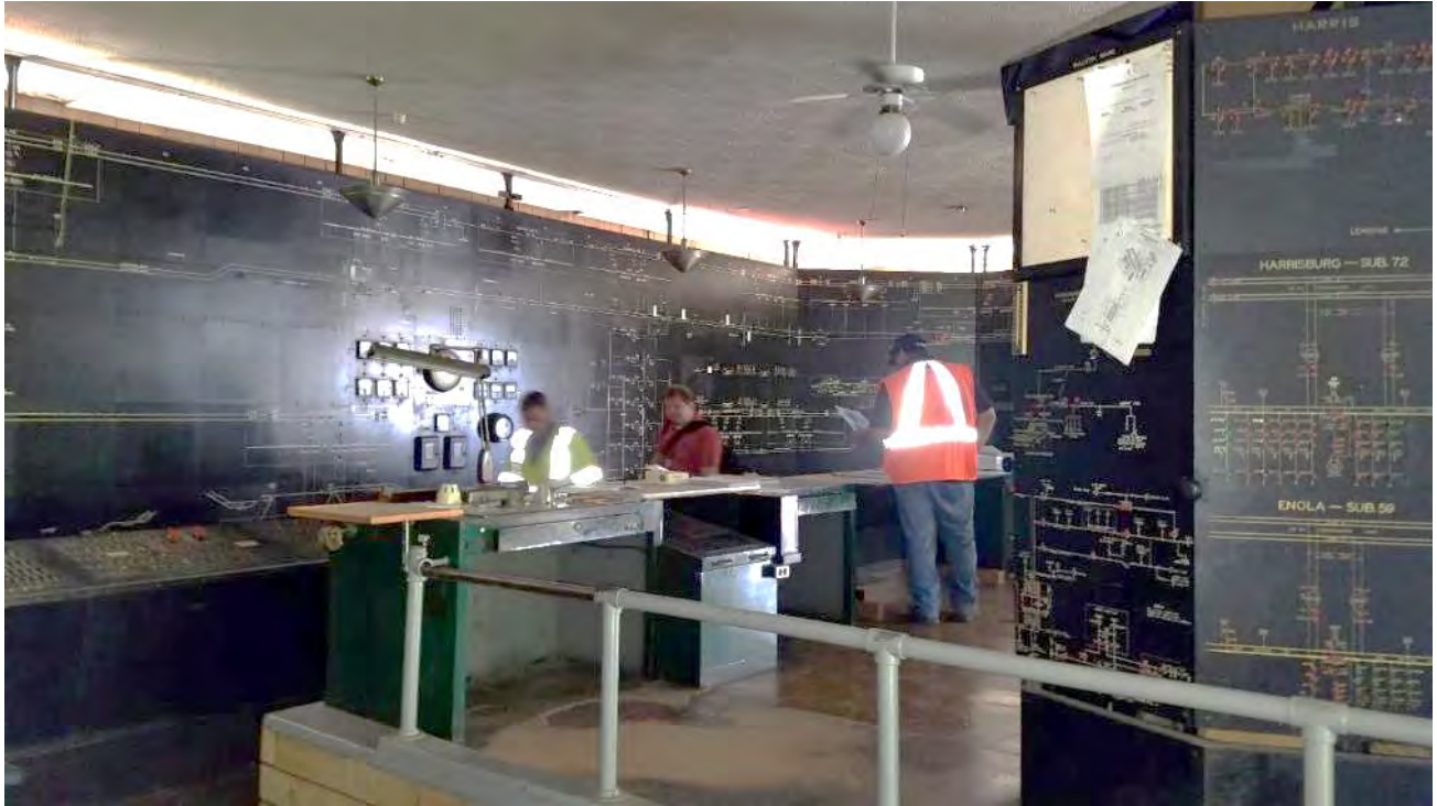
Image 31: Interior view of power directors room, second floor, 2017.
