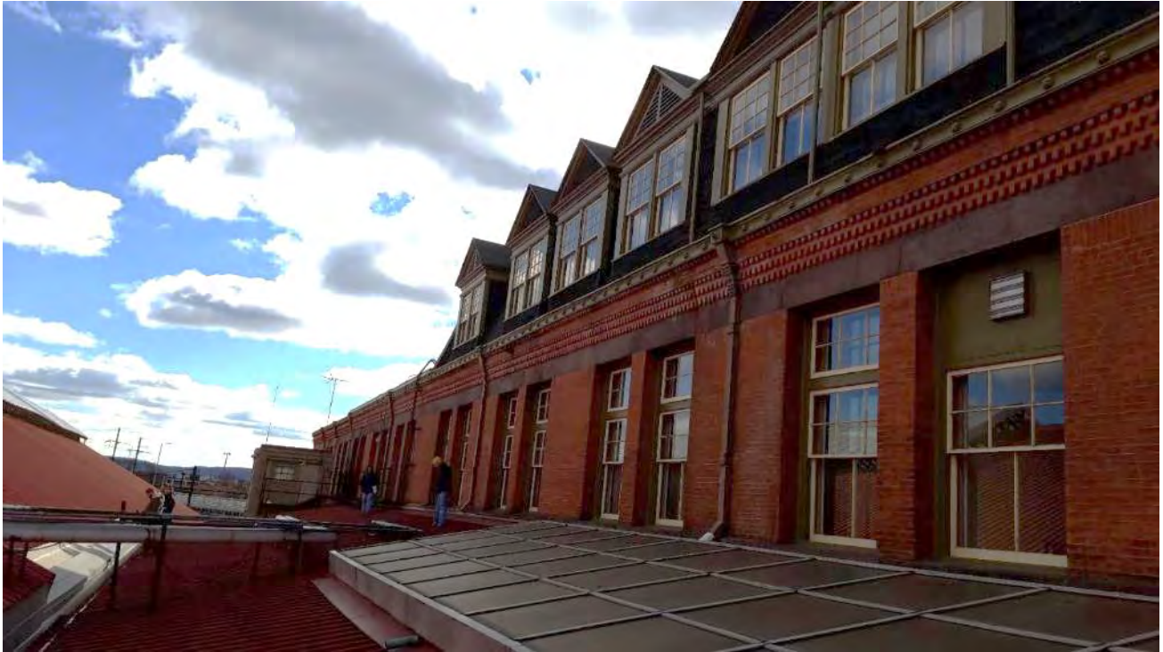
Image 41: View from roof of rear (east) elevation looking south, showing second and third stories of original section, 2017.
