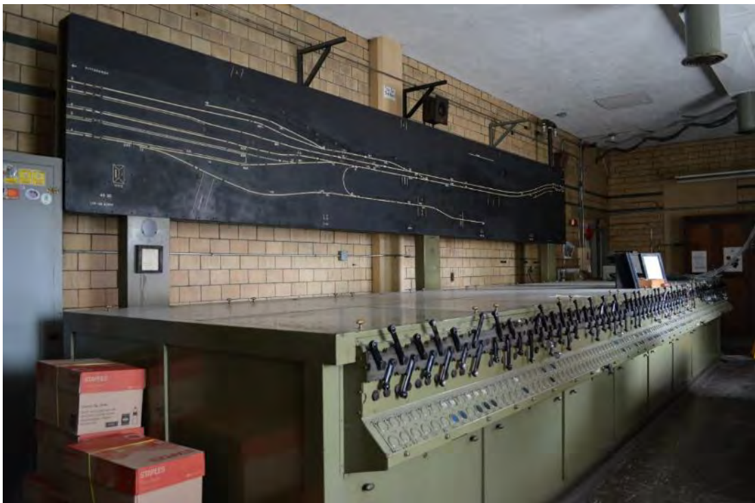
Photograph 39: View of interlocking equipment, first floor of the 1937 addition, looking northeast.
