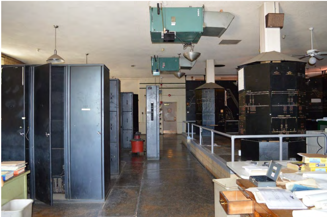
Photograph 14: Five rows of General Electric equipment cabinets (left).
