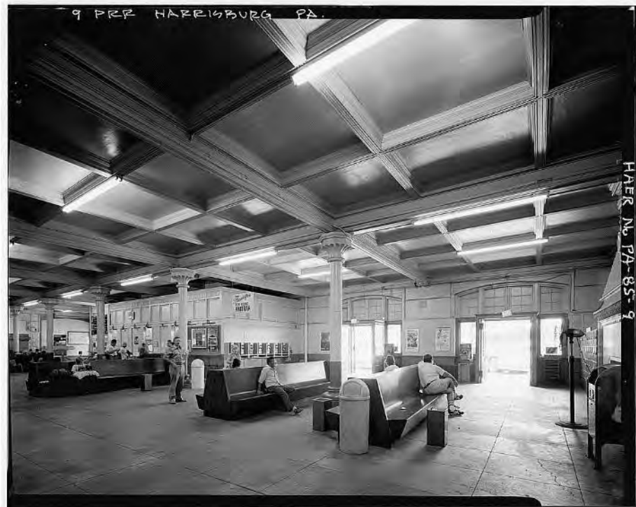
Image 13: View, looking southwest of main lobby, first floor, showing front entrances and ticket booth. Note wooden beam ceiling and cast-iron columns. (HAER 1985)
