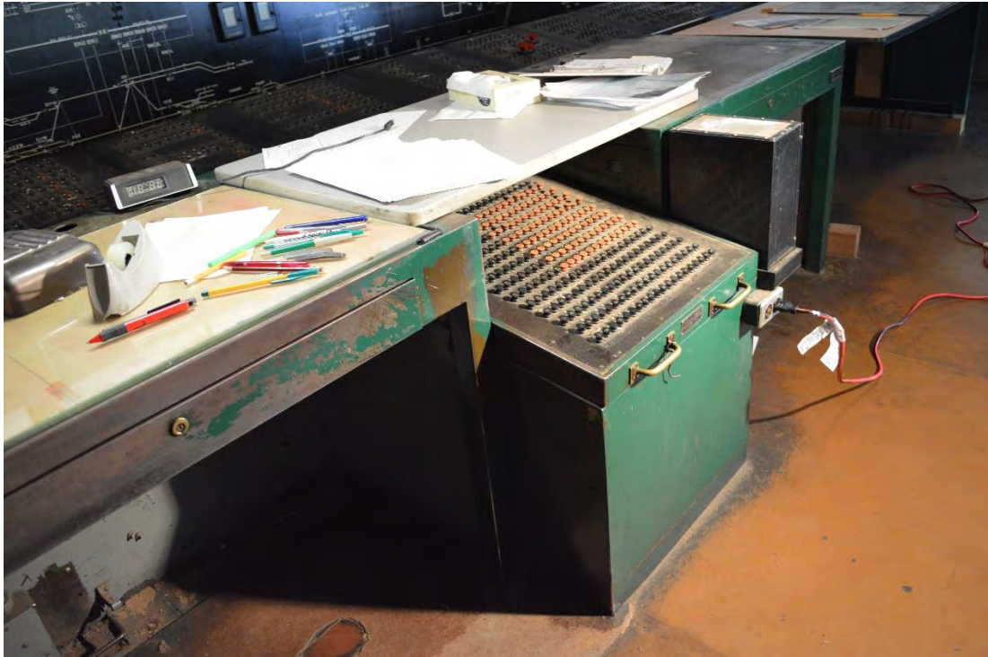
Photograph 13: Detail of Kellogg Switchboard & Supply Co. signal control unit.
