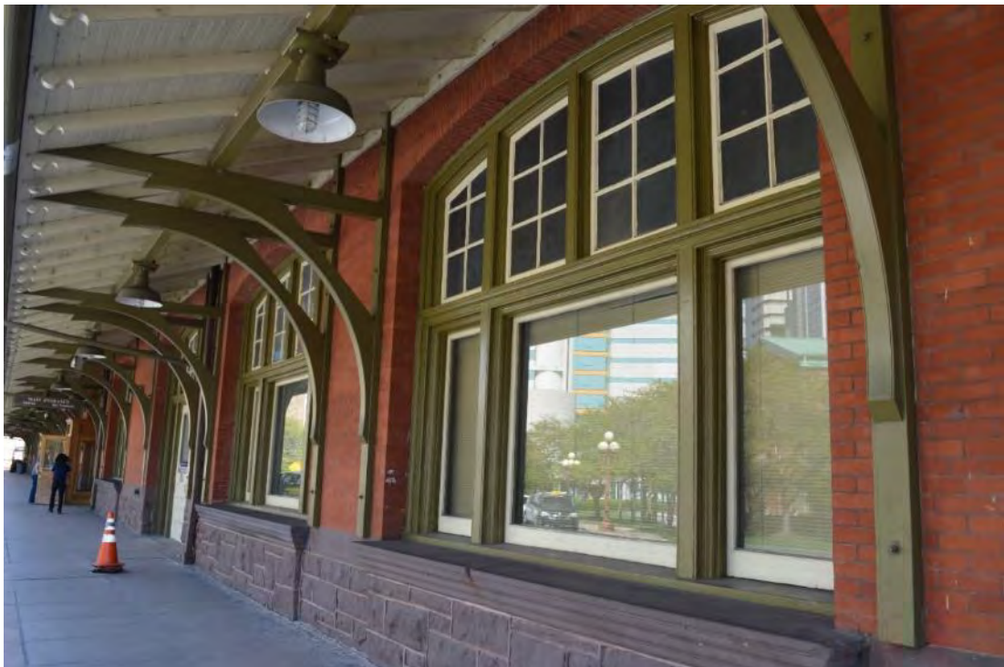
Photograph 10: Detail of passenger station facade showing first story windows and canopy support brackets, looking north-northeast. Note the brownstone watertable.
