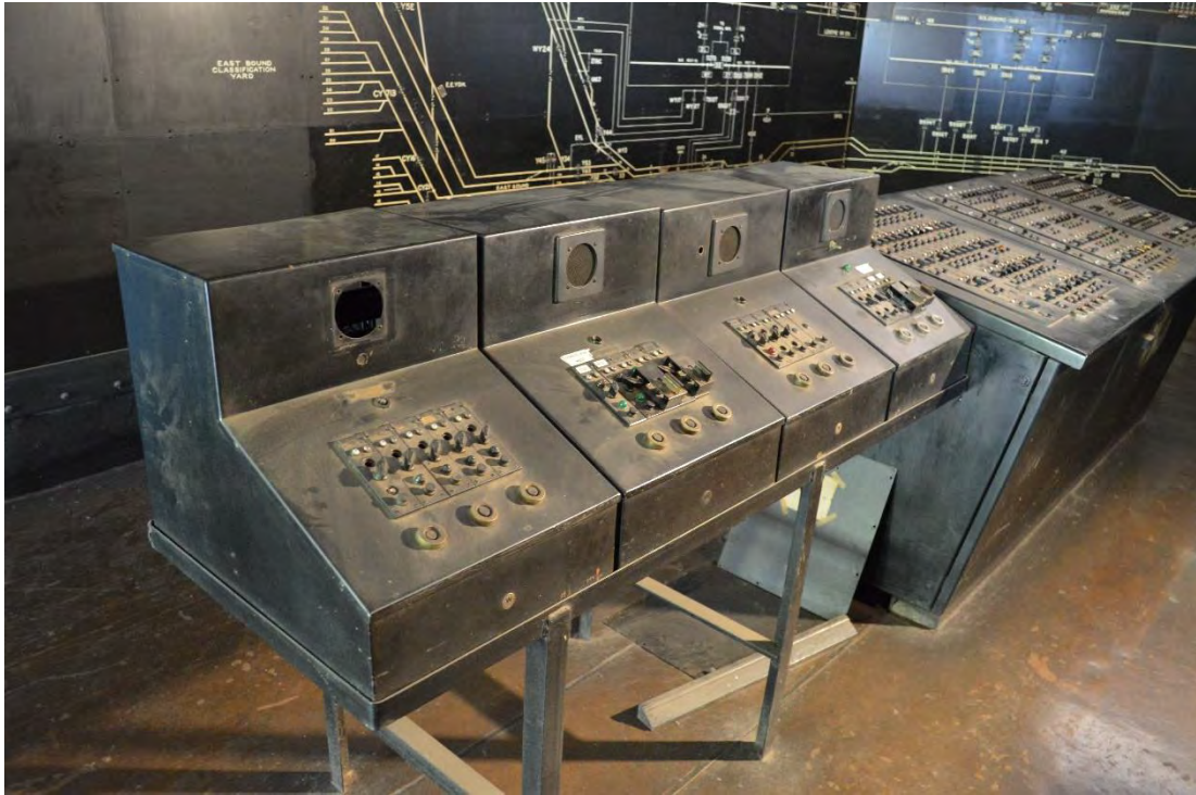
Photograph 11: Westinghouse Polaricode JR console.
