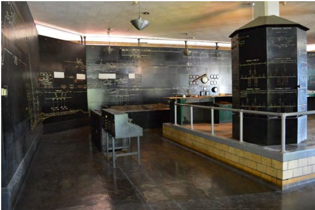
Photograph 43: View of Power Director's Room, second floor of passenger station, looking north.
