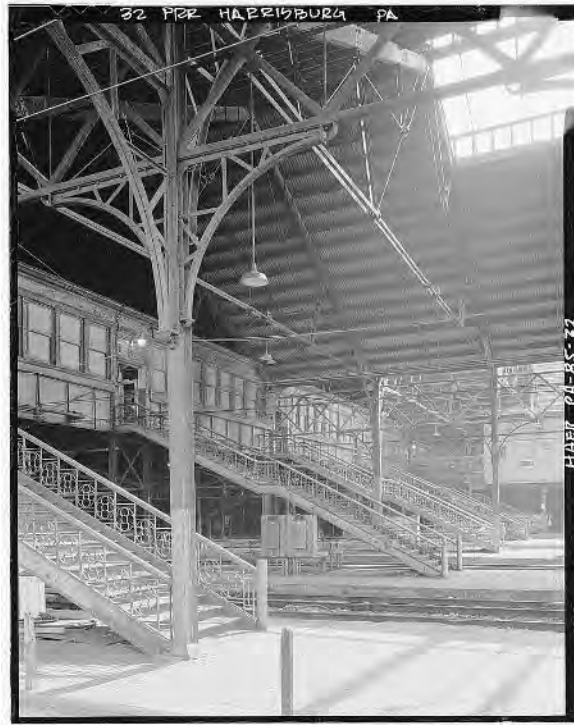
Image 35: Oblique view of concourse (north side), plaza level, looking toward station building, showing passenger access stairs. Note typical shed column brackets. (HAER 1985)
