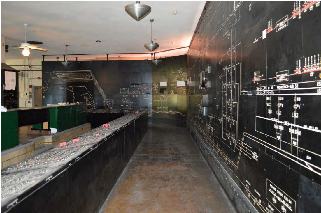
Photograph 1: General Electric Model Board.
