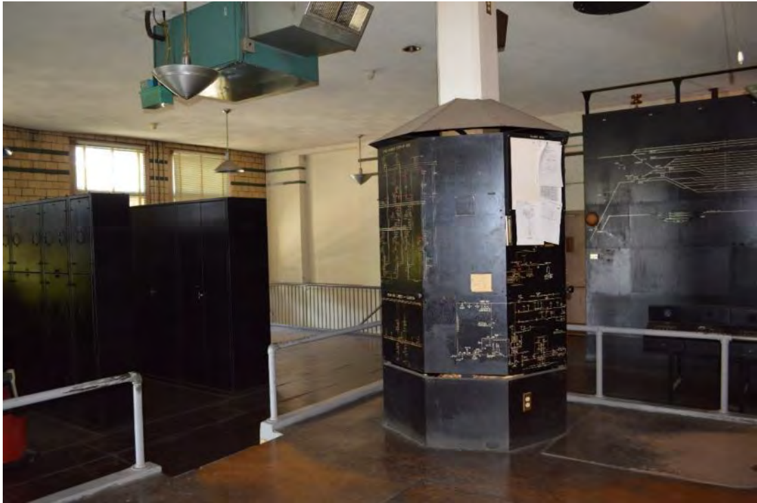
Photograph 42: View of Power Director's Room, second floor of passenger station, looking northwest.
