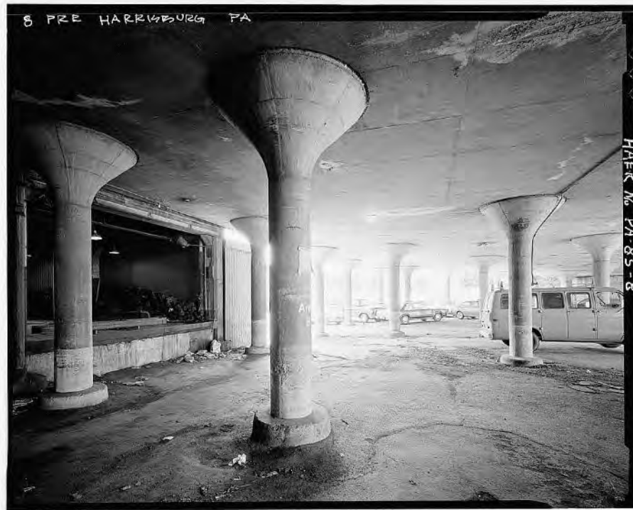
Image 11: View under viaduct at south end of station building, showing staff parking area and loading dock. (HAER 1985)
